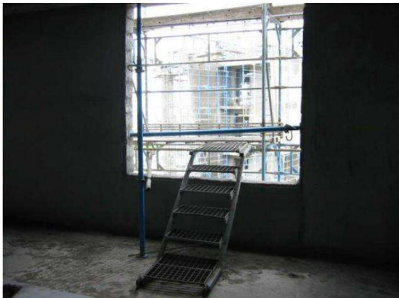
Proper Access to workplatform
